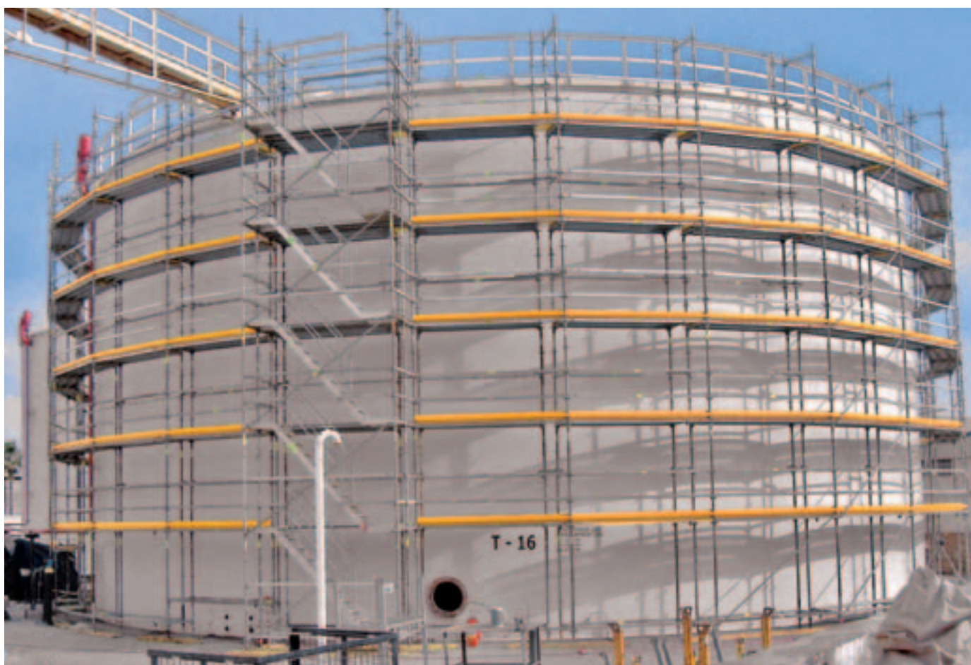
Circular container scaffolded with a three-part side protection complete with system components.
