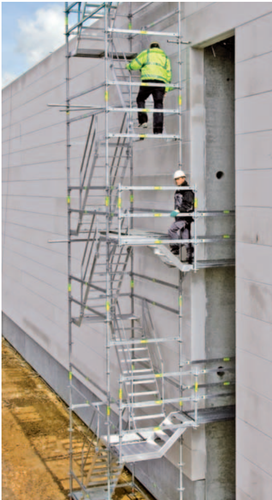
Height adjustments on building openings are installed independent of the floor height.
